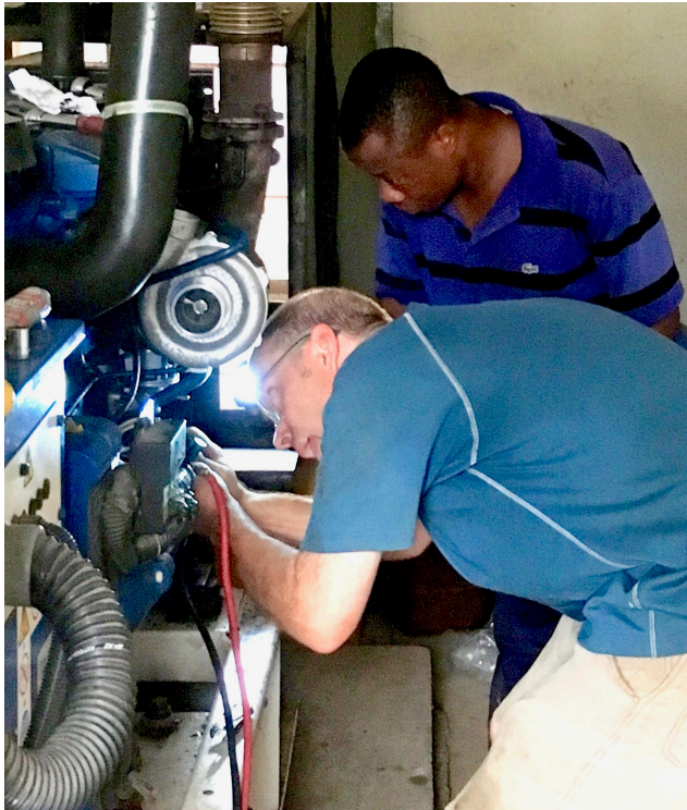
Scott has been learning a lot about running and maintaining a large generator. Here he is installing a new turbo charger.
