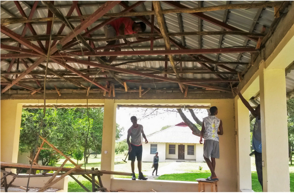
Rafiki youth renovating the gazebo. Look closely—there are five kids in this picture!
