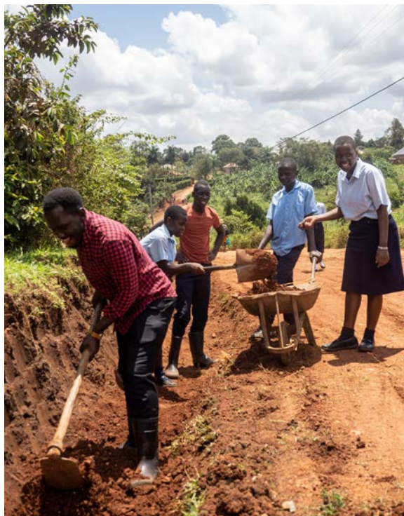
Headmaster Assistant Derrick leads students in a service project improving the drainage on the road outside the Village
